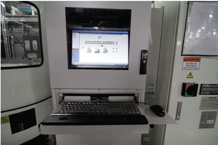
The MAS-A5 controller features a direct link from the line to the tooling department for instantaneous transfer and storage of all tool data.
